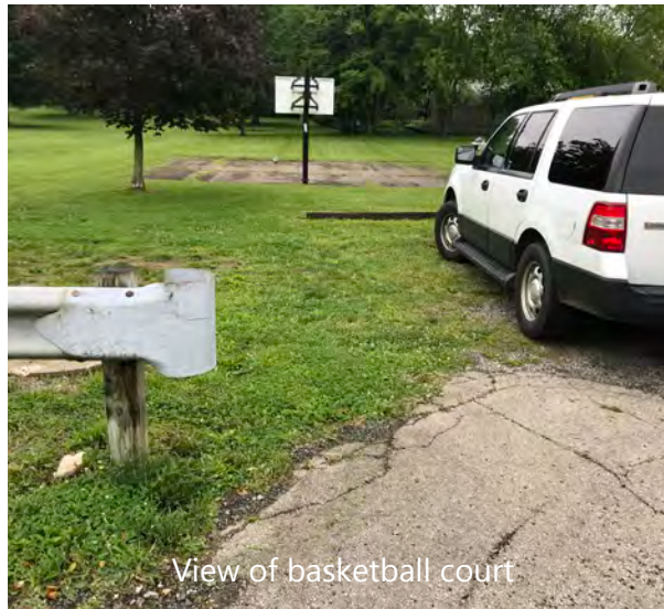
View of grass taking over parking lot
